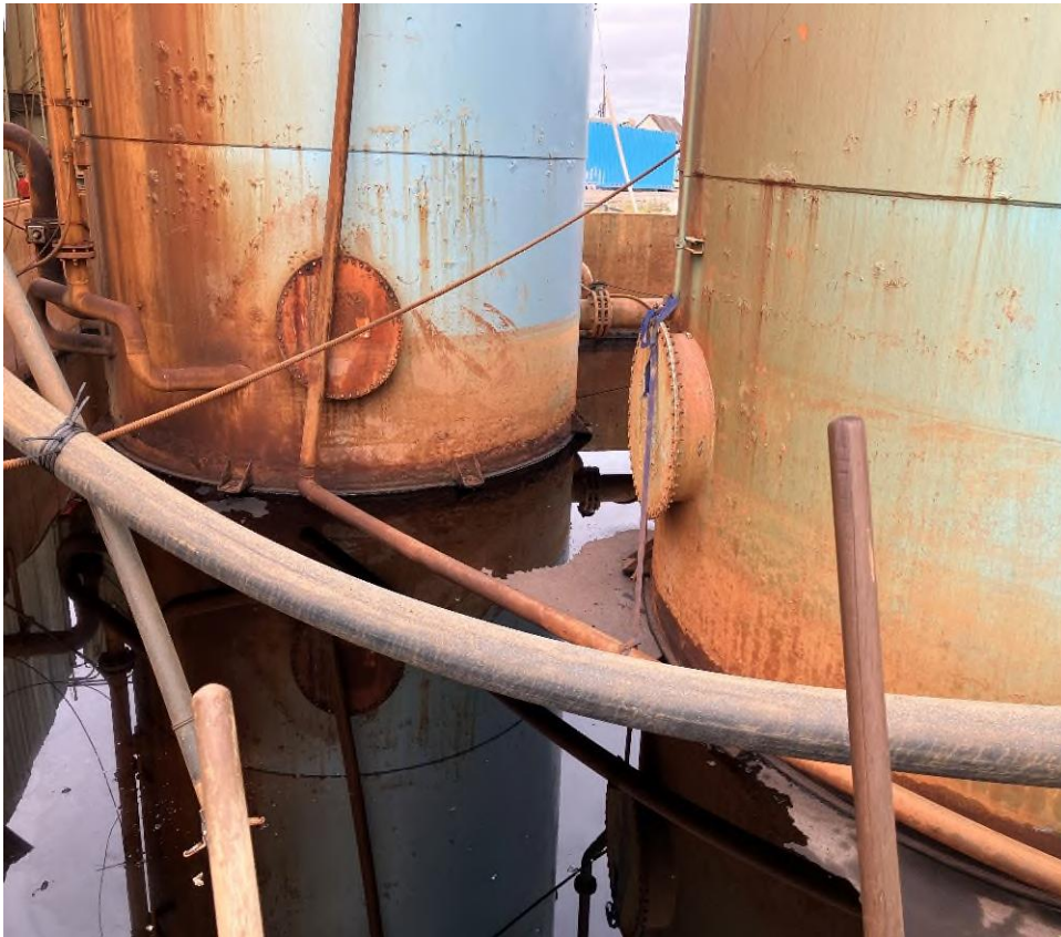
Photo Number: 10 Date: 8-7-2024 Comments: Picture of leachate release that occurred within the AST secondary containment.
