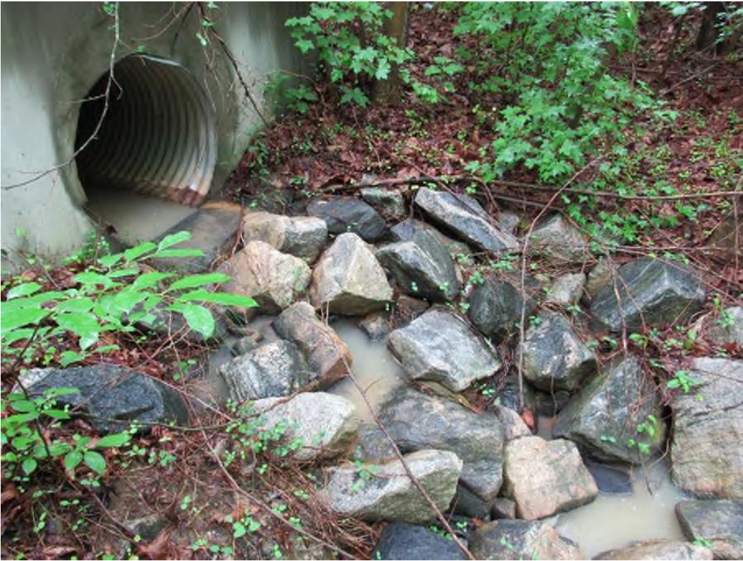
Site Name: Shoosmith SLF Permit# SWP587 Taken By: Jeremy Kazio and Andrew Peal Page 8 Photo Number: 15 Date: 6/16/2025 Comments: Active discharge from VPDES permitted outfall serving SB-12
