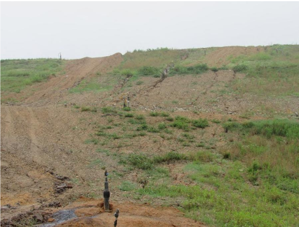
Photo Number: 24 Date: 6/16/2025 Comments: Example of excessive rilling (and leachate seep)
