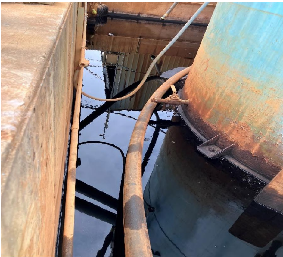
Photo Number: 12 Date: 8-7-2024 Comments: Picture of leachate release that occurred within the AST secondary containment.
